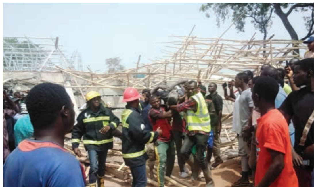
■ Rescue operation at the site of the collapsed building
