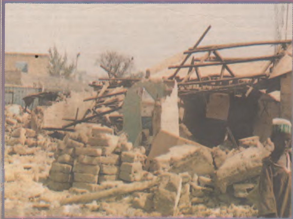
Demolished structures along the Nyanya-Keffi road.
