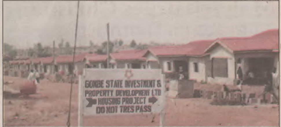
50 unit 3-bedroom housing complex currently under construction in Gombe to ease accommodation problem.
