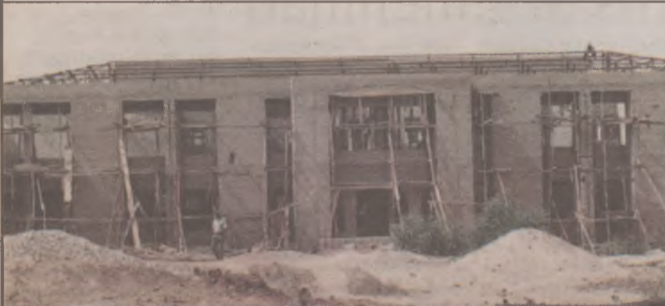
The deputy governor's office under construction in Gombe, one of the projects embarked upon this year.
