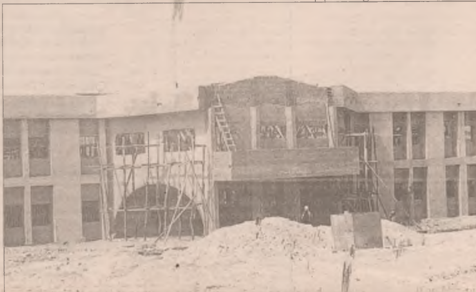
A building under construction. An expert says that it could last 40 years if properly managed.
