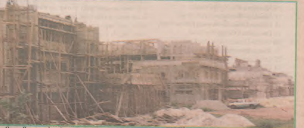
Imo State Secretariat Complex under construction at New Owerri, along Owerri - P/Harcourt Road
