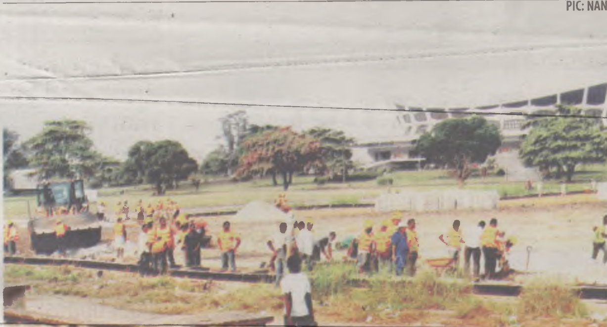
CONSTRUCTION work on the Okokomaiko/CMS light train project in progress beside the National Theatre, Lagos, yesterday.
