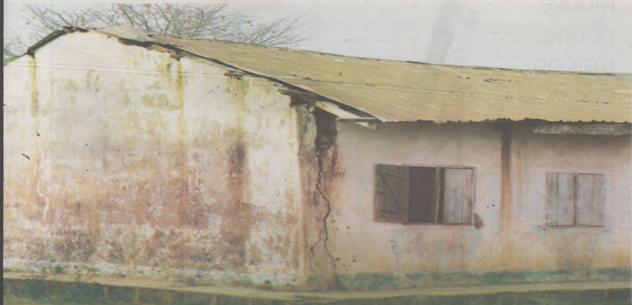
Deerless looking school in Abocho: Apart from lack of power supply in the area, there is no pipe borne water, poor roads, no chalk, few or no blackboards and poorly motivated teachers.
