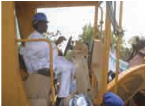
Gov. Mai Mala Buni flagging off the construction of Potiskum township road
