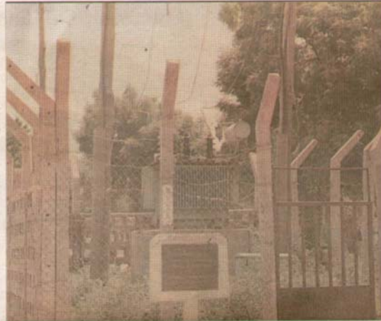
Main transformer built organised by the community.
