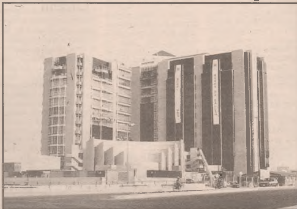
The new Central Bank of Nigeria headquarters, Central District Abuja, under construction.
