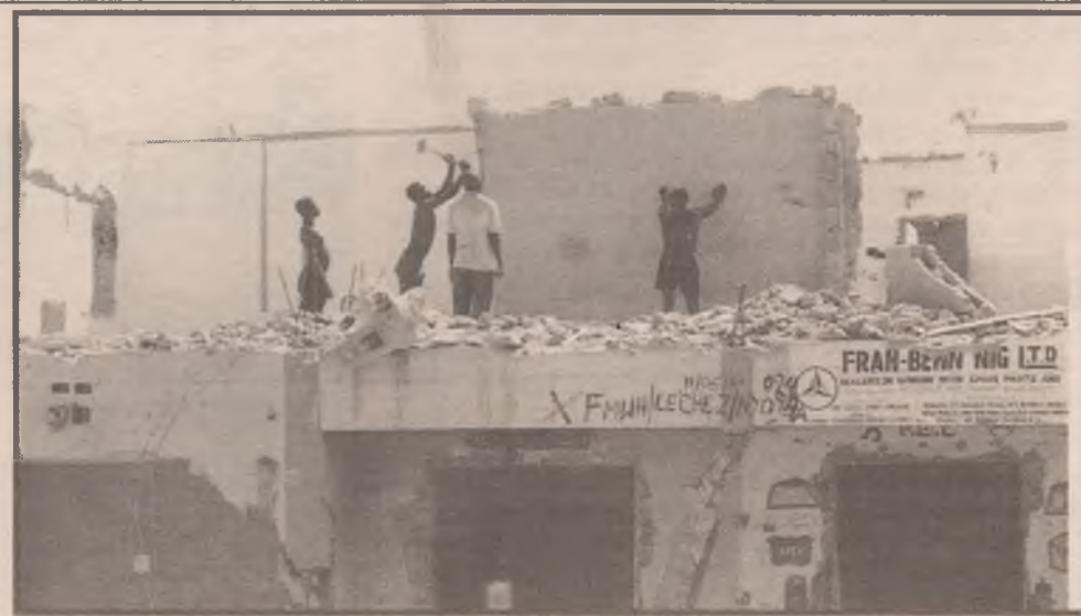
A demolished property in Nyanya, to make way for the Abuja - Keffi dualisation project
