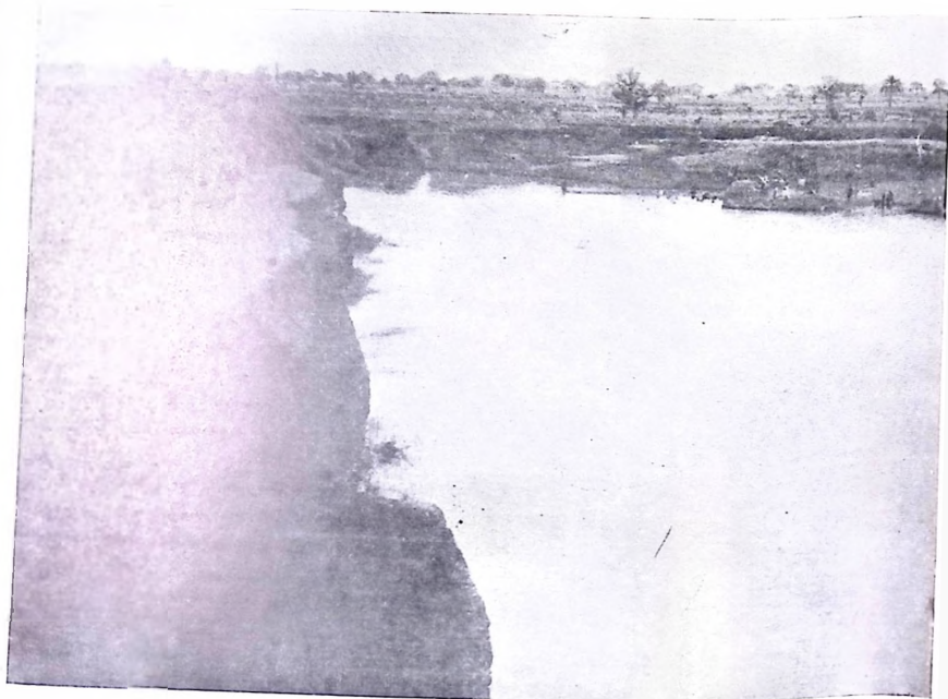
Borrow-pits at Mile 3 Challawa Road, showing imminent collapse of Wall
