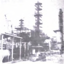
A Section of the New Port Harcourt Refinery set under construction. Part of the Port Harcourt Refining Company Ltd.
