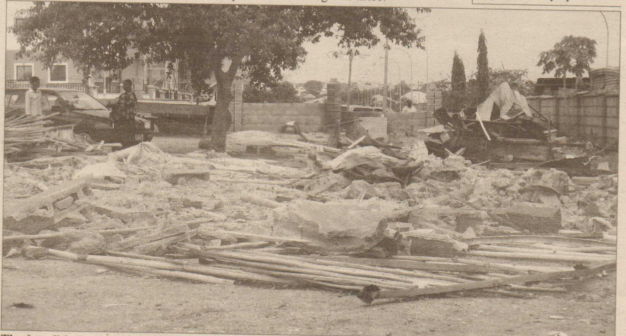
The demolished structures at NUJ Abuja Council premises at Utako yesterday.
