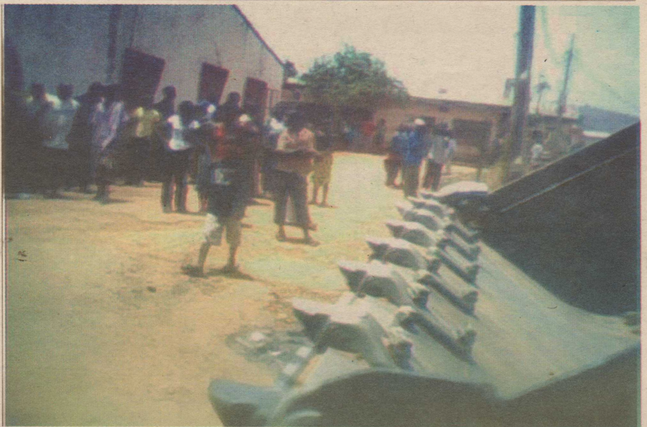
Karu residents staring in anxiety at a bulldozer ready to commence demolition.
