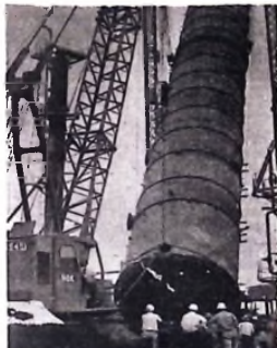
An 80-ton steel which forms part of oil Refinery structure in Alasa Elemo, Port Harcourt.
