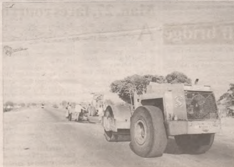
The main thoroughfare of Yola road leading to Kurmi market under construction.
