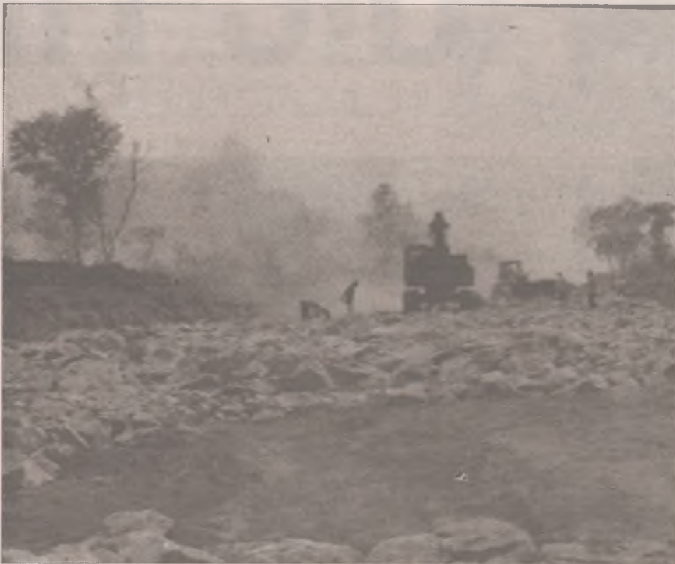
Road construction work progressing on the Kuje satellite town development scheme in Kuje area council, Abuja.
