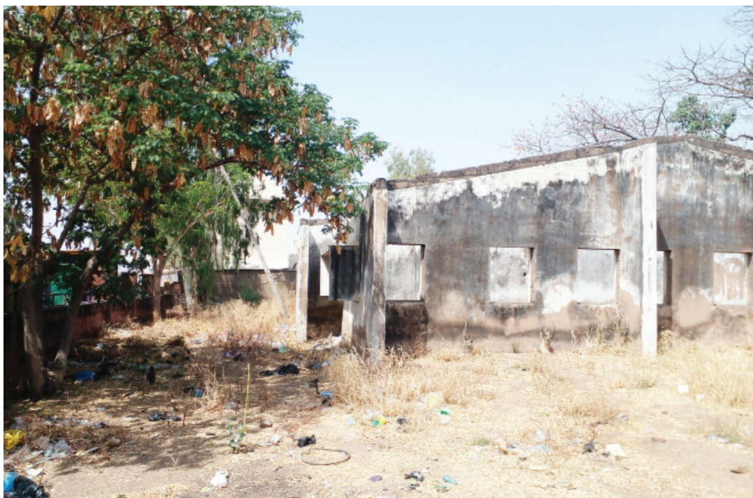
■ Taraba state Library building located along Hammaruwa road Jalingo which was razed down by mid night fire in 2009 and was renovated PHOTO: Magaji Isa Hunkuyi
