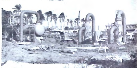
• Egbin gas plant, and (inset) Mines and Power Minister Sheriff Musa. Uninterrupted power supply?
