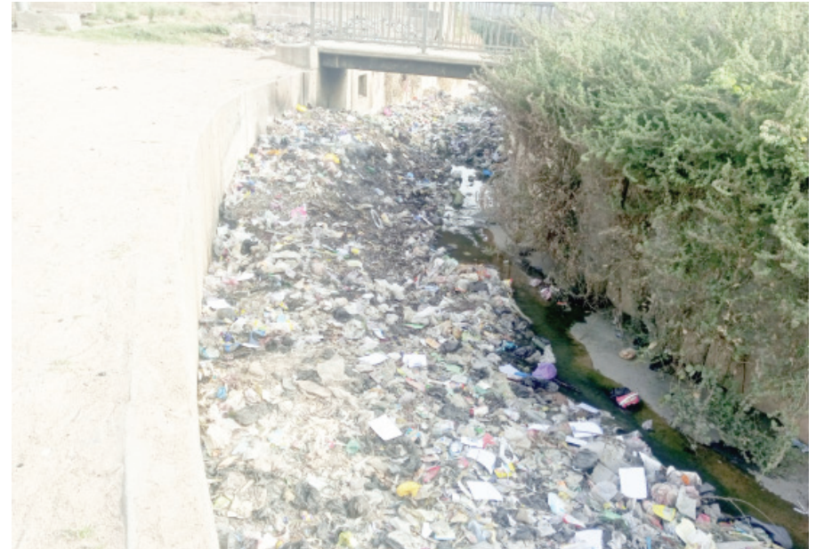
Julius Beggar drainage filled with refuse dumps and human feces behind Oceanic Bank, Mobil Roundabout, Minna
