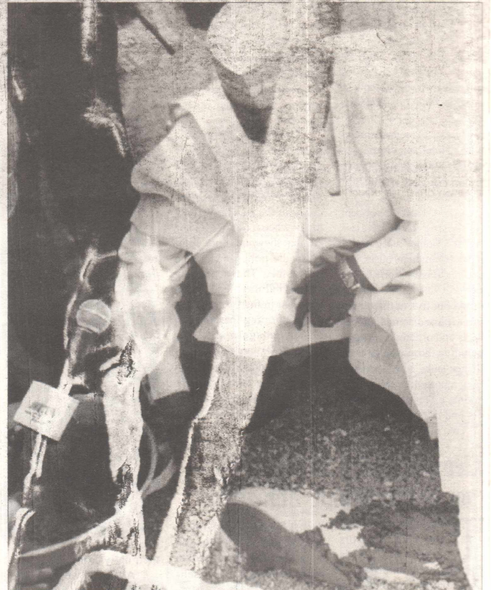
Governor Shekarau doing official foundation laying of the new Tamburawa water treatment plant.
