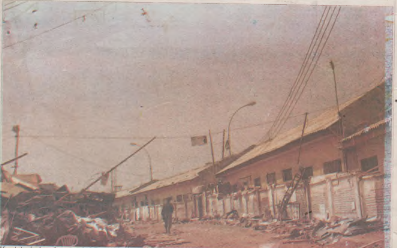
Mangled container-shops detached from the approved shops by AEPB.
