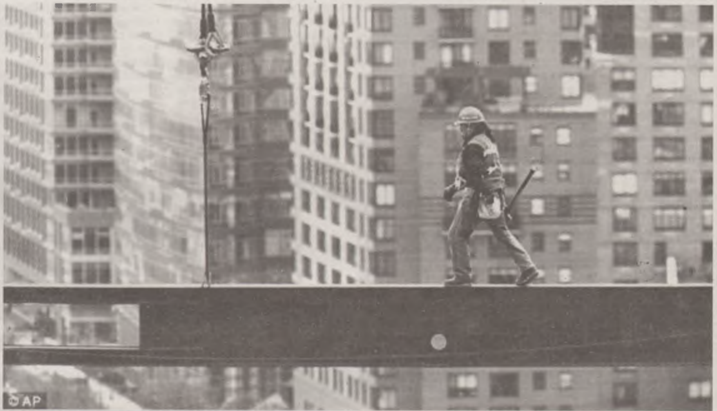
AN ironworker walks on a beam at One World Trade Center construction site in New York at the weekend.
