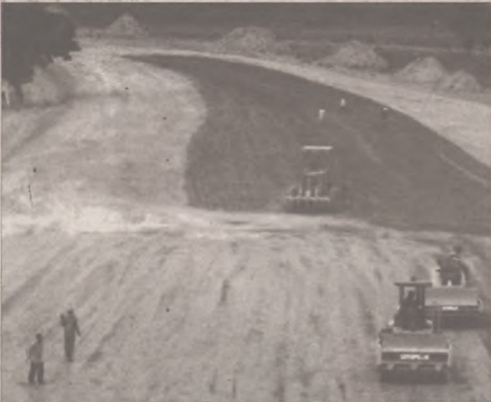
A view of the Kaduna Eastern by-pass road project delayed by lack of funds
