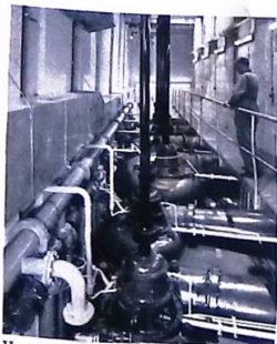
Vertical screw pumps in a sewage pumping station at Geneva, Switzerland. Total delivery 70 000 m 3 /h (257 000 gpm).
