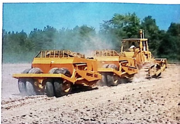
Cat D6D SA Tractor pulling Rome scrapers for heavy duty levelling. Fast, low-cost means of handling soil displacement.
