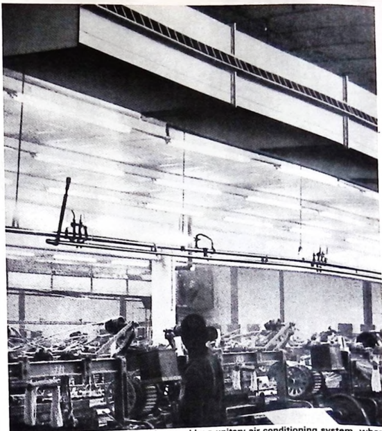
This weaving shed in a textile mill is served by a unitary air conditioning system, where individual self-contained plants are supplemented by direct injection of moisture vapour by compressed air and water sprays. The service pipework and spray heads for this equipment can be seen above the looms. This shed is maintained at 80 per cent relative humidity.
