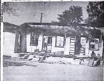
• Dasuki's house destroyed during the riot.
