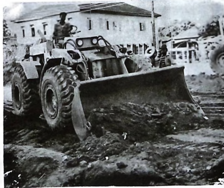
Road construction in progress. Listen to Spotlight On Federal Government projects - Friday, 16.15
