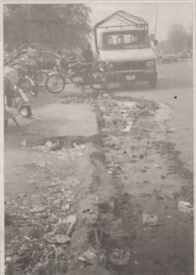
Despite Kano government's effort to clear drainages of waste, many waterways are still blocked at Fagge along Murtala Muhammed Way. Pix: Musa Kazaure
