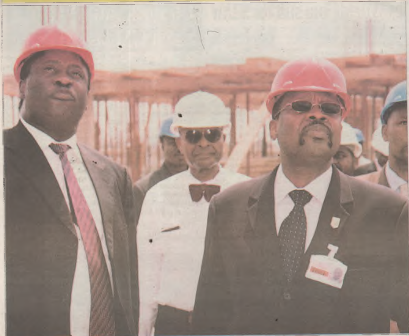
L-R: Mr Wale Babalakin, Chairman, Stabilini Visiononi and Managing Director of the Federal Airports Authority of Nigeria (FAAN), Engineer Mohammed Gambo Umar, while inspecting the reconstruction of the burnt terminal of the Murtala Mohammed International Airport, Lagos ...recently.
