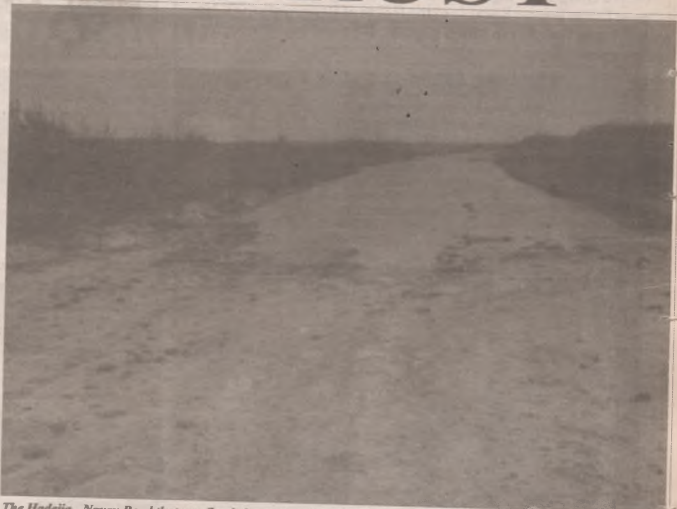
The Hadejia - Nguru Road that was flooded by waters from the Wetland irrigation scheme. Pix: Musa Kazaure
