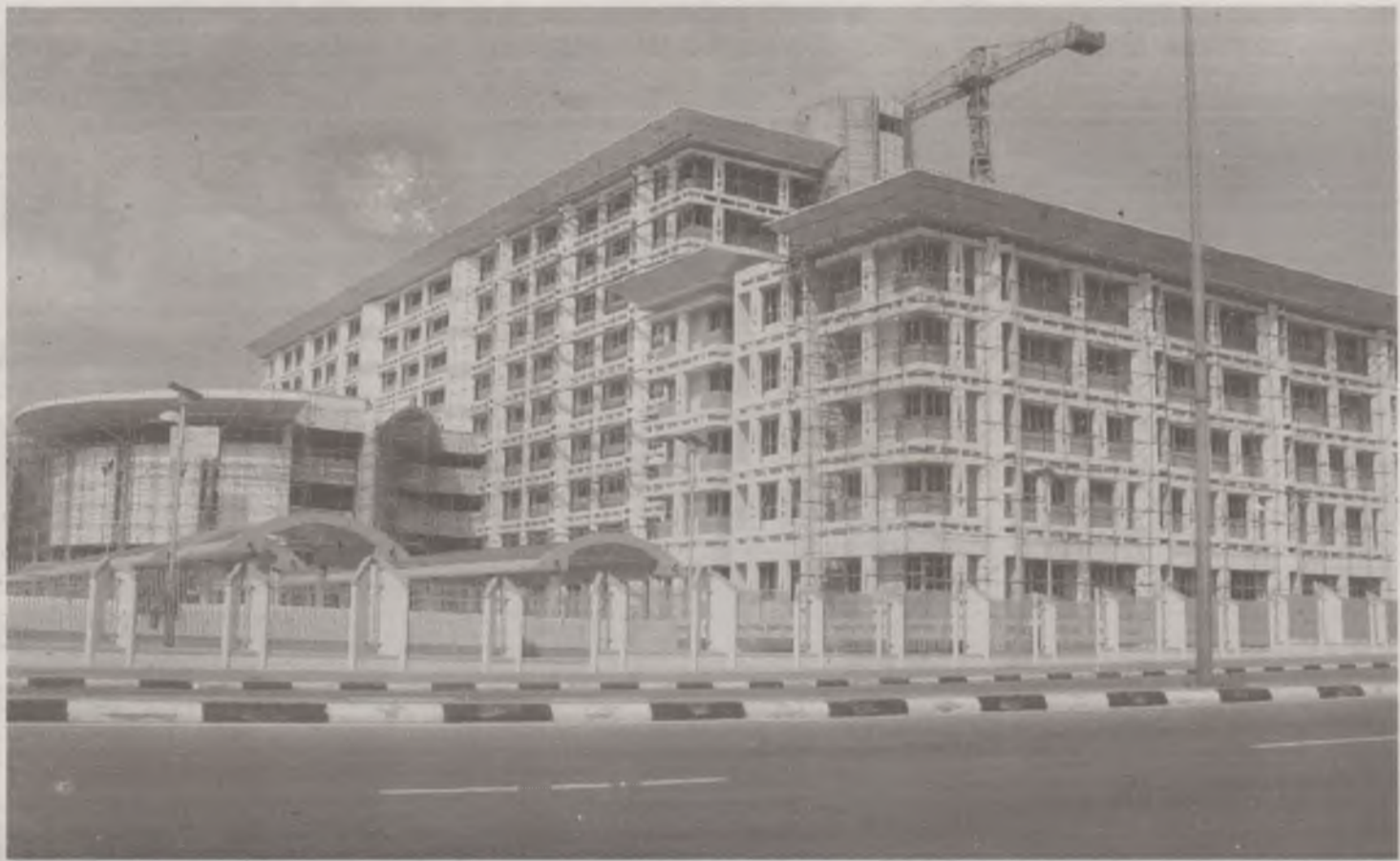
THE Federal Ministry of Foreign Affairs Headquarters, nearing completion in the Central Area, Abuja
