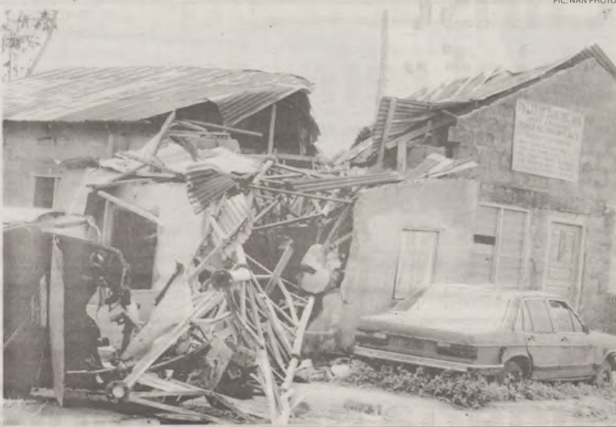
A communication mast that damaged a church building after a rainstorm in Eket yesterday.
