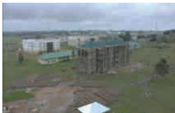
More infrastructure work being carried out by the Lalong Rescue Administration in PLASU Bokkos
