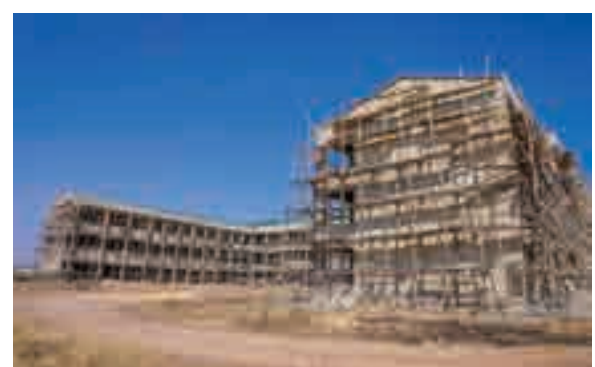
One of the new Faculties under construction at the Plateau State University Bokkos
