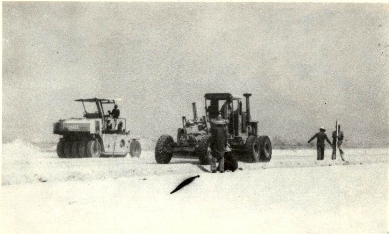
Spreading and compacting of sub-base material of the Maiduguri Airport in progress
