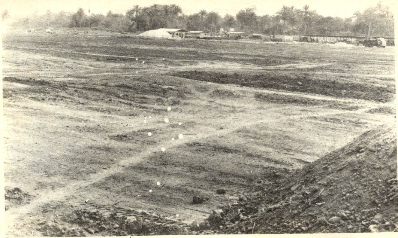
Topsoil strip of the main apron from the new Port Harcourt Airport under preparation
