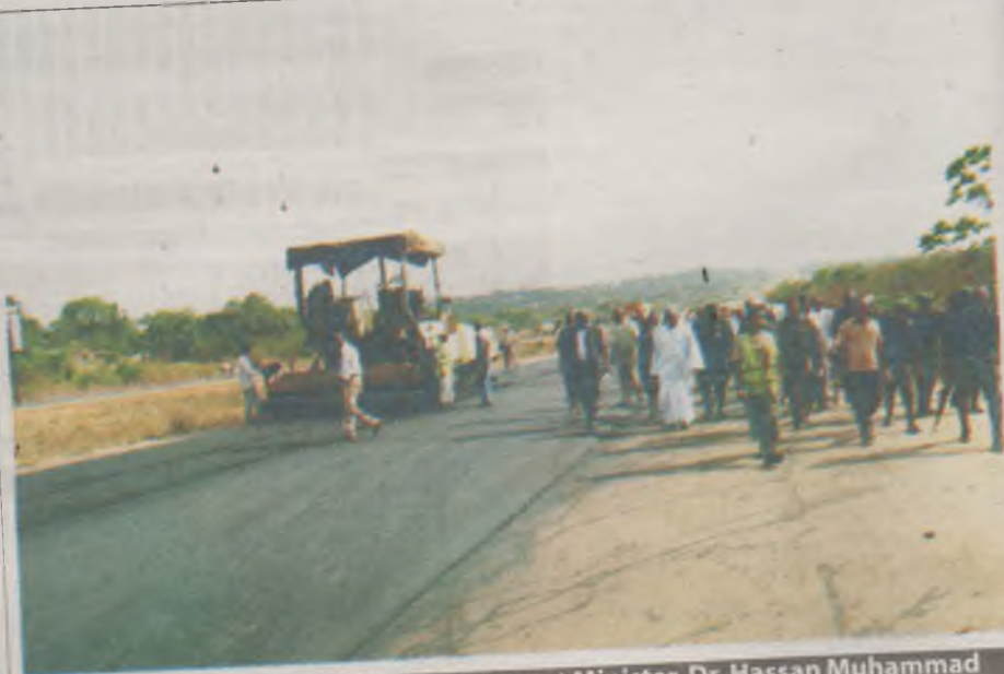
WORKS, Housing and Urban Development Minister, Dr. Hassan Muhammad Lawal, inspecting on-going rehabilitation works on the Enugu - Port Harcourt dual carriageway last Thursday
