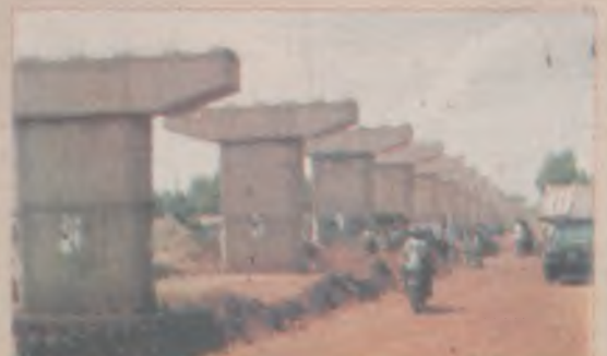
The first ever Sokoto fly-over which is costing the State Government Billions of naira is an effort worthy of commendation.
