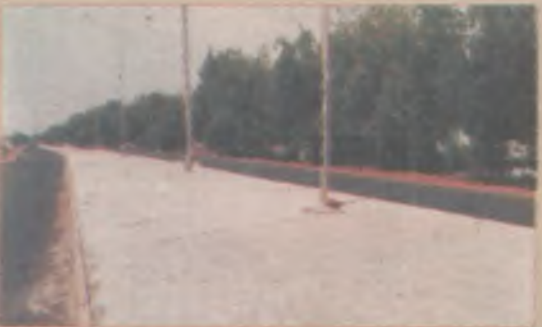
The interlocking works on Sokoto- Kano road almost completed under the Sokoto State Government beautification project.
