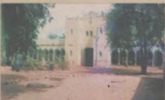
The old Nagarta College Sokoto established in 1905 by the then colonial masters under going serious renovation.
