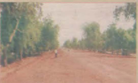
Dualisation of a 3km Garba Duba township road also in completion stage.
