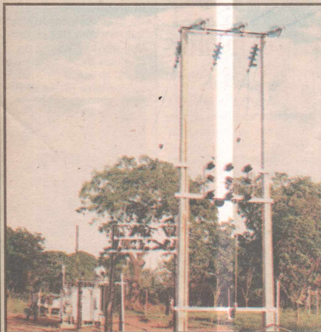
Adikpo Electricity Project (Kwande Local Government)
