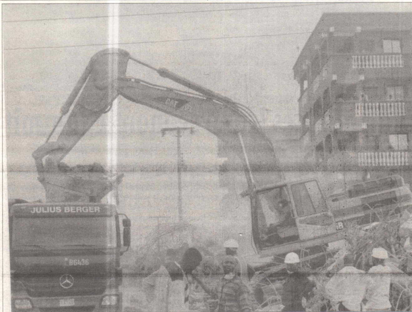
A payloader clearing the debris of the collapsed building at Amukoko Area of Lagos...recently
