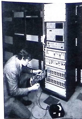
Adjusting low two panels of an audio channel on the Plessey PRD 1650 multiplex unit.
