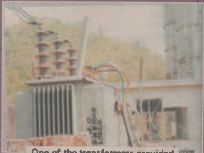
One of the transformers provided for rural electrification
