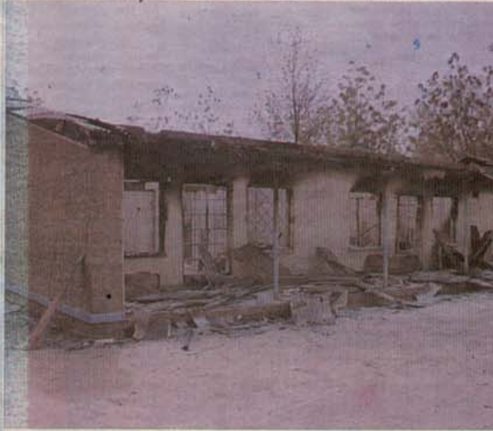
BUK staff quarters burnt during the Yelwa Shendam reprisal violence in Kano
