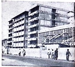
Near the Connaught Hospital, buildings for the new training centre for nurses are now well advanced. The cost is being met partly by the government and partly by the US AHEAD Foundation.
