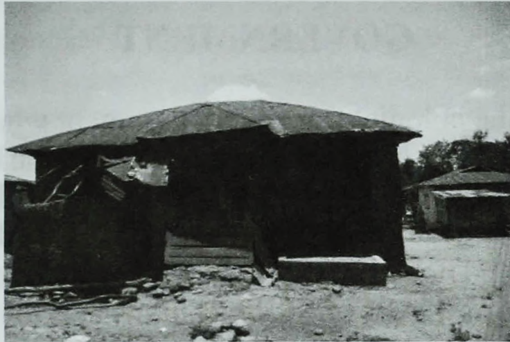
The house built by Olukotun Aso now dilapidated.
