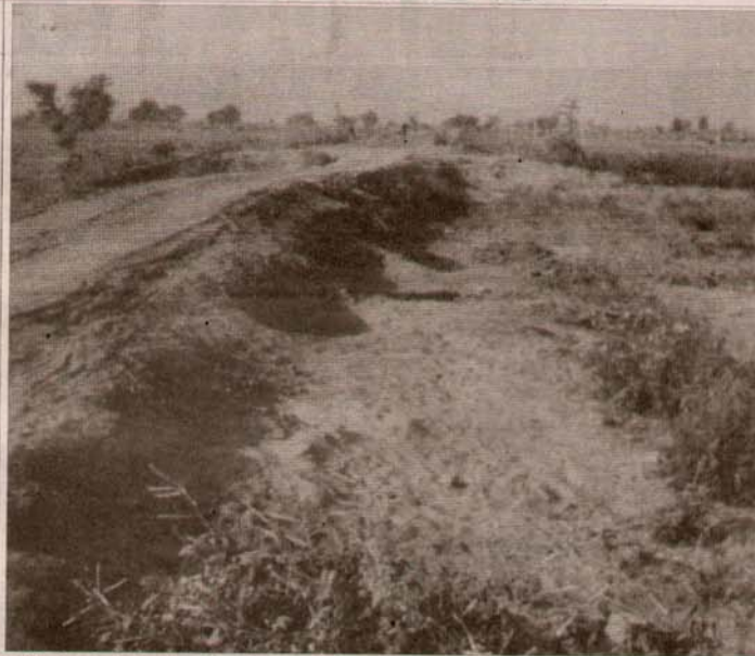
Problem of erosion in Jigawa State. Jahau-Gujungu road under erosion threat.
