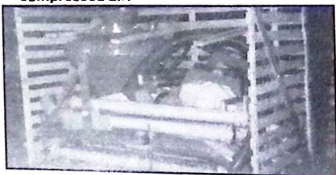
An SEM pump from Crow Hamilton Ltd. producing constant flow by means of compressed air.
