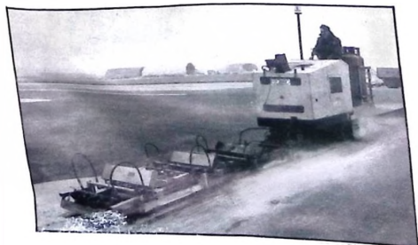
Joad's Superplane cuts asphalt to a depth of 50mm. in a single pass.
