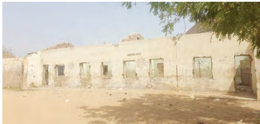
■ One of the structures at GSS Kwakwachi to be renovated through the PPP arrangement
