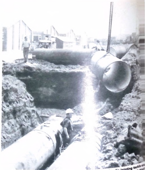
The Stantyte joint coupled with the use of the efficient hydraulic jointing tackle maintains a high laying rate to the twin 1100 mm diameter rising sewerage mains being laid below ground.
