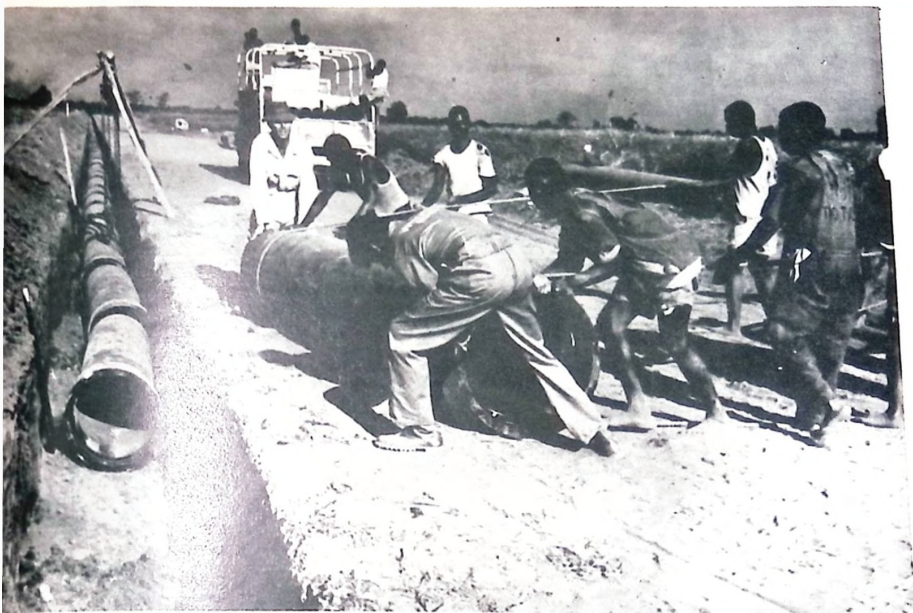
Local labour being employed to lay TAC's pipes for a drainage scheme
