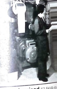
Containerised 62.5kVA standby set North Sea oil rigs.
