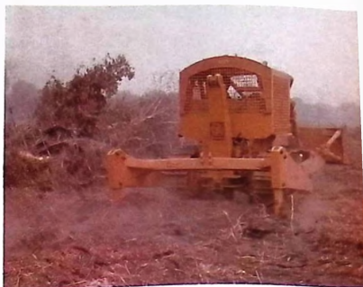
D7G Tractor with Fleco Root Plow as demonstrated at T & E seminar 'Operation Land Development'
