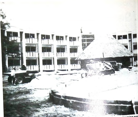
General view of construction under way at the site, with restaurant wing, swimming pool in the foreground, and thatched bar between.
