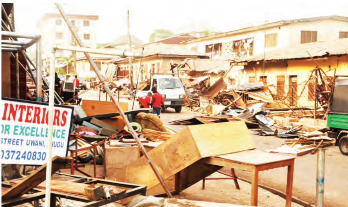
■ Illegal structures demolished along Bishop Aniofu Furniture Makers Business Areas in Uwan, Enugu yesterday
