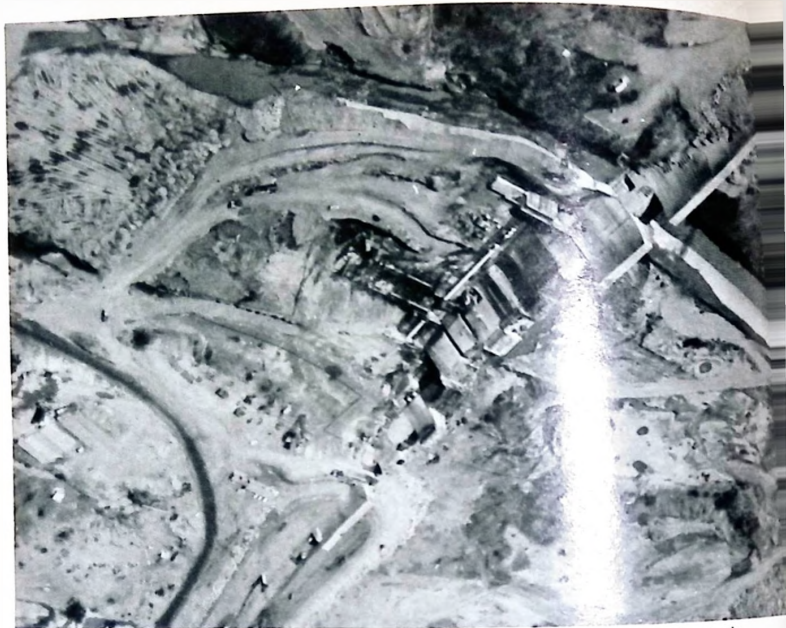
An aerial view of the Bakolori Dam, still under construction in the Sokoto-Rima river basin.
