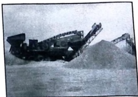
A 36 x 30 Goliath mobile primary plant from Goodwin Barsby is crushing and screening gravel for aggregate.
